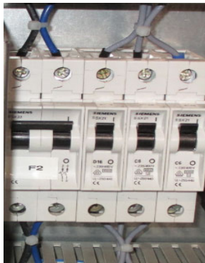
primary and secondary fuses
